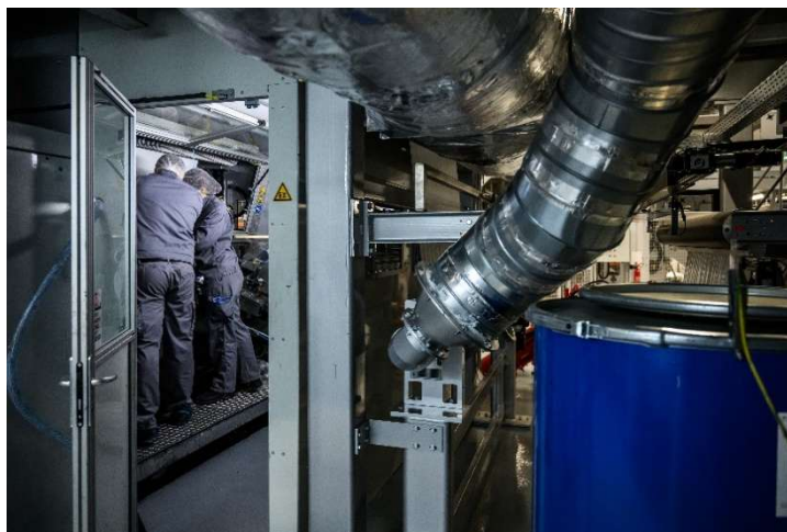
Figure 21 Coating line at the Chenôve facility and fume extraction system
