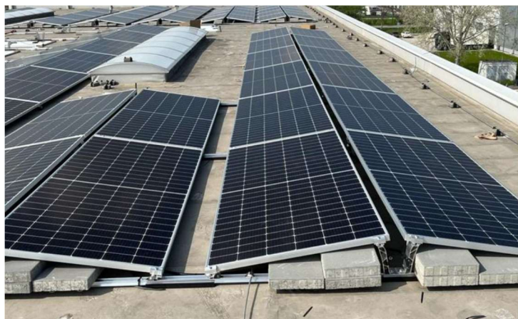
Figure 17 The roof equipped in 2023 with solar panels at our Senec plant in Slovakia
